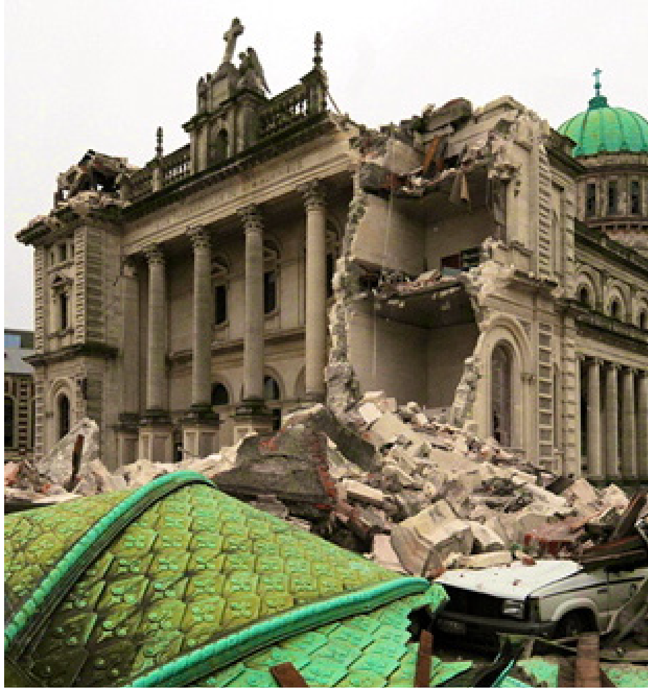
A prominent Christchurch landmark lay in ruins after the devastating magnitude 6.3 earthquake in New Zealand Feb. 22. Hundreds died and hundreds of thousands are in dire need. Photo courtesy of Brenda Knight.
